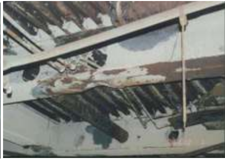
(b) Local buckling of the steel beam
