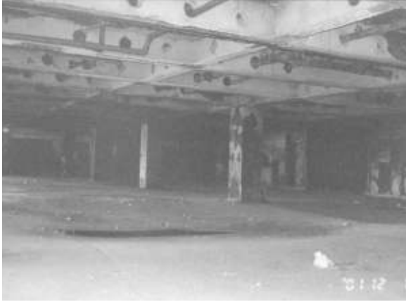
Fig. 9.9 Large deflection of the slab in a building after fire attack
