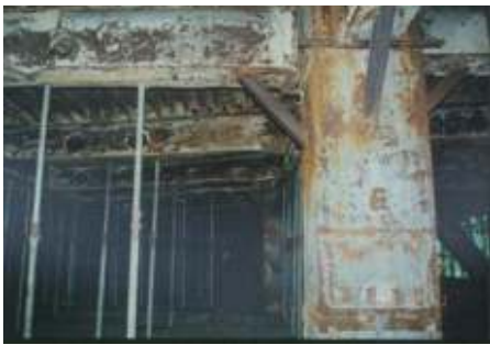
(a) Fracture of the beam-to-column connection
