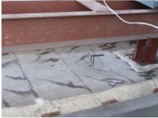
Fig. 7.39 Water exudes through cracks in the slab in the test CB150 (mm)
