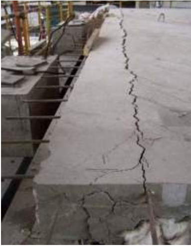
Fig. 9.19 Cracks along the long edge on S-1
