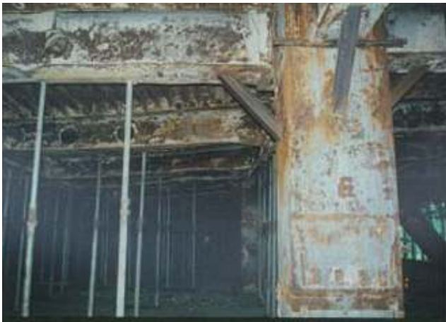
Fig. 7.18 Damage to the beam-column connection by a fire
