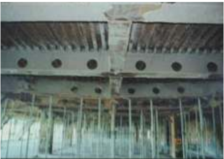
(c) Large deflection in the steel beam
