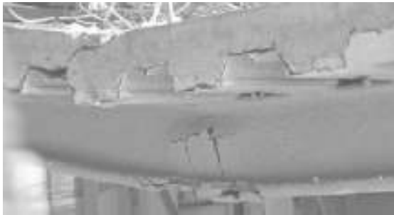
Fig. 5.11 Failure of the composite beam
