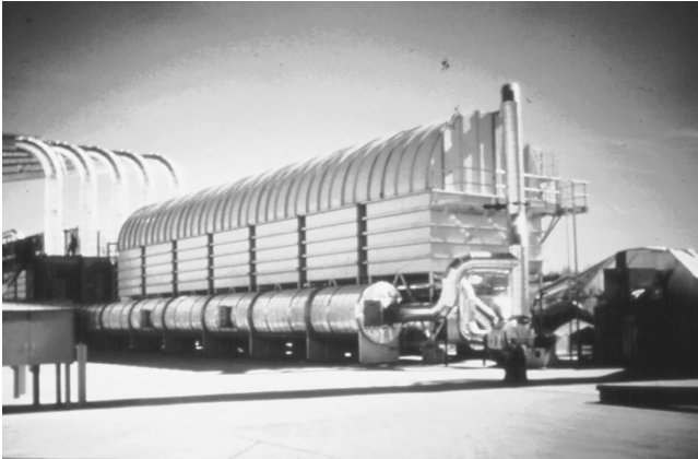
FIGURE 13.12 Seven-chamber regenerative thermal oxidizer. (Courtesy of Smith Environmental Corp.)
