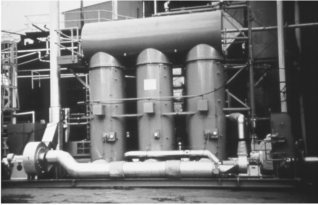
FIGURE 13.11 Small three-chamber regenerative thermal oxidizer. (Courtesy of Smith Environmental Corp.)
