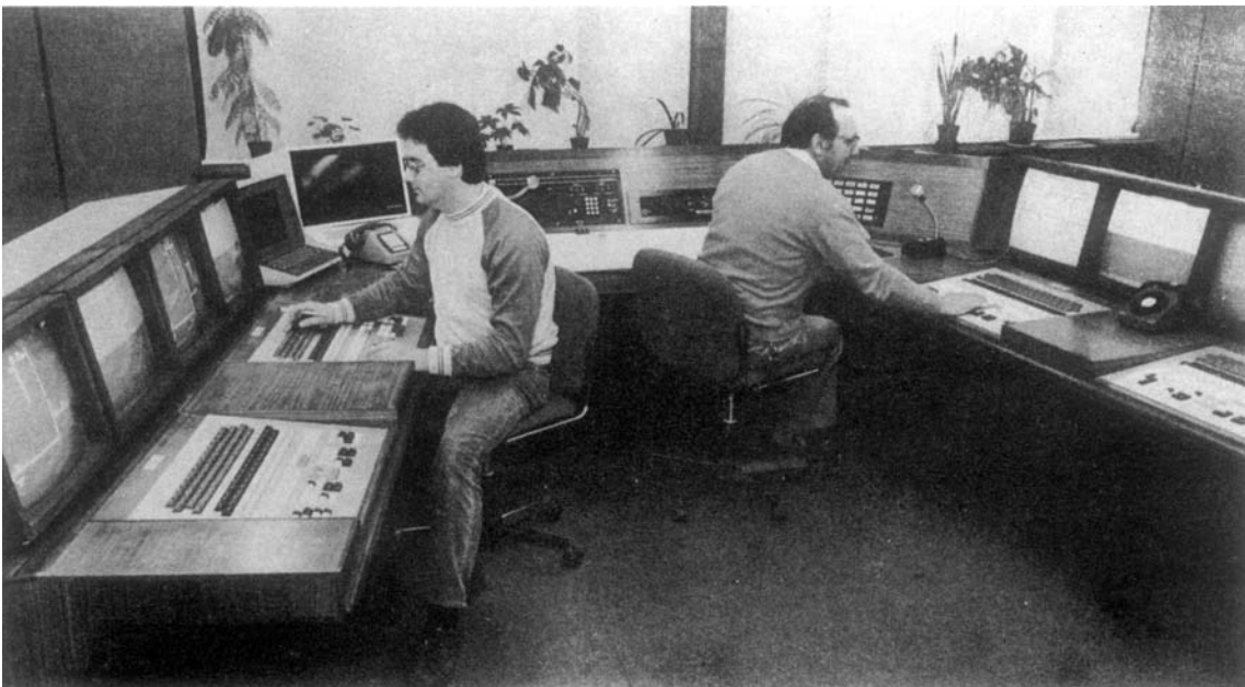
Figure 48.28 A surface control room
